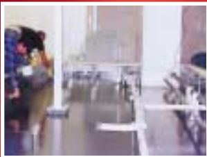
A bund floor in this electronics factory protected against possible hydrofluoric acid leaks with two coats of Chemi-Tech UC.
